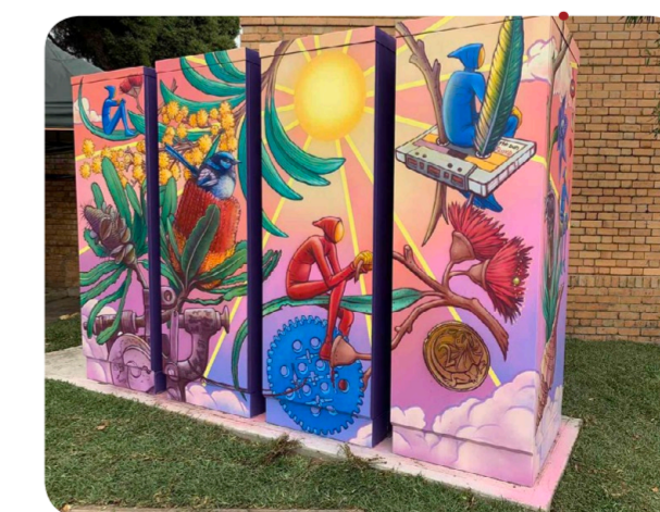
Energy storage in Melbourne. Source: OneStepOffTheGrid / Brant Kozlovskis
